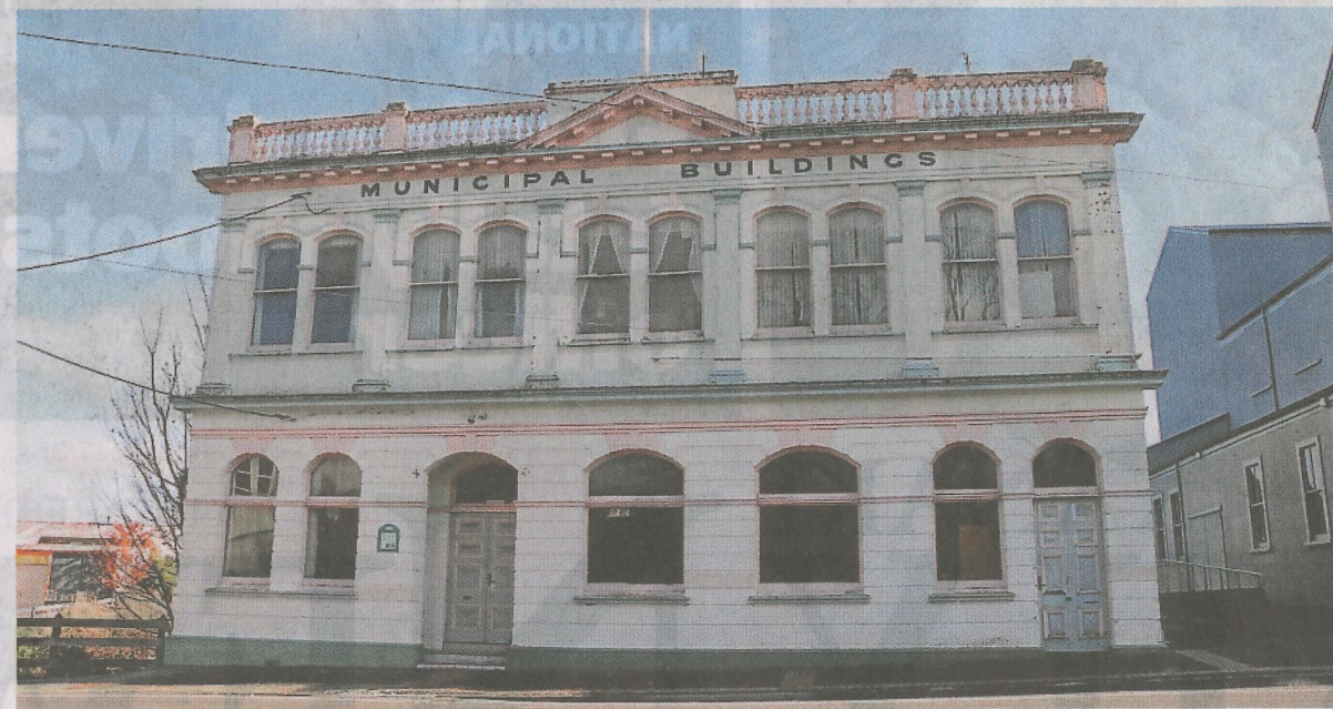
The former Eltham Borough Council building, which needs major repairs and earthquake strengthening, is already attracting interest from possible buyers.
