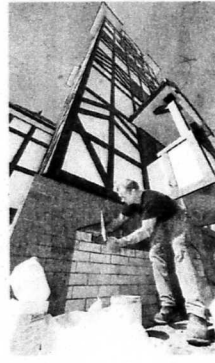
SET: Bricklayer Jim McIntee puts the final touches to the clock tower base.
