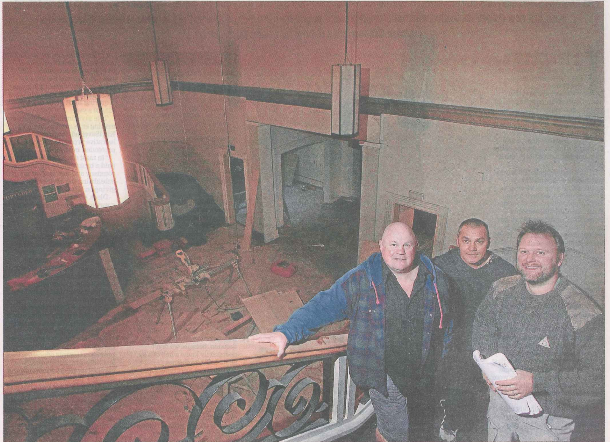
Big job: Doc van Praagh, left, Dave Haskell and Kymon Hill say it will cost hundreds of thousands of dollars and take six weeks to renovate the Mayfair in New Plymouth and turn it into one of the city's largest hospitality ventures. Photo: CAMERON BURNELL/FAIRFAX NZ
