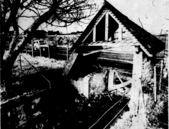
BELOW: One of the last visible reminders to motorists on Devon Rd that St Luke's Anglican Church was once here... a memorial lychgate, built in 1914. It came to grief recently during a car accident, although steps are being taken to see if it can be repaired.
