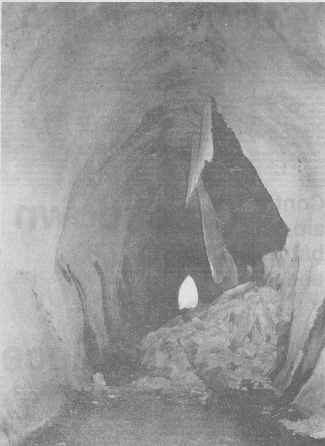
Tangahoe Valley Rd tunnel will be blocked at both ends after tonnes of earth caved in through the gunite lining, blocking access to Lake Rotorangi.
