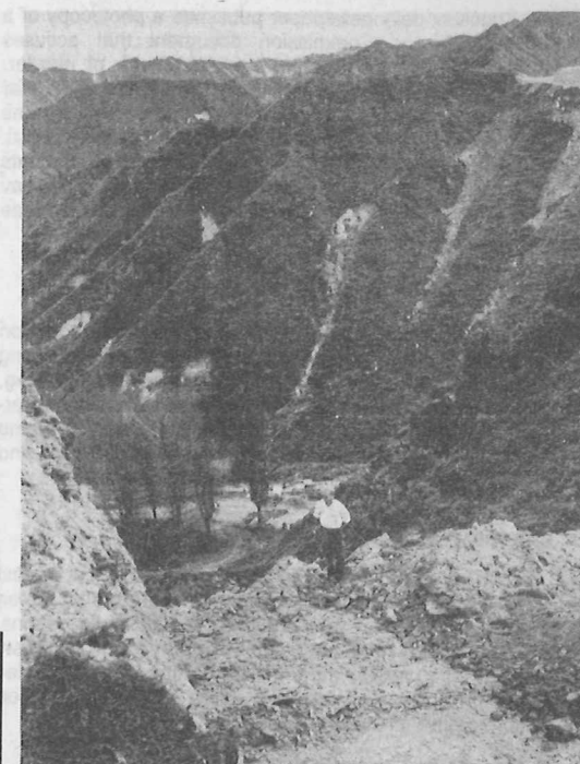
Hawera District Council engineering assistant Gordon Campbell is overseeing a new route to Lake Rotorangi being cut 40m deep through this ridge to one side of the collapsed tunnel. The road will slope gently through the gully pictured, to rejoin Tangahoe Valley Rd beyond the tunnel.
