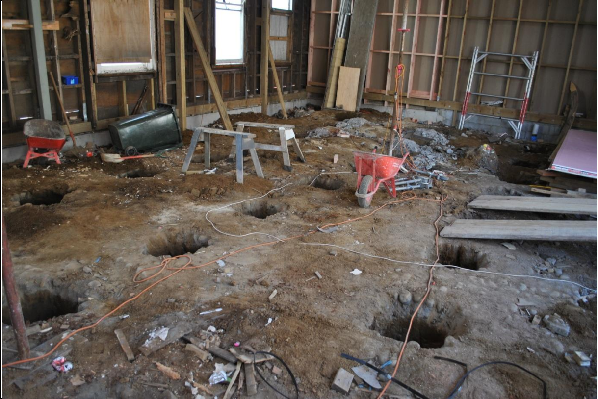
Plate 21: New pile holes cut through the cobbles; the extent of earthworks undertaken below the cobbled area below the former Messenger extension
