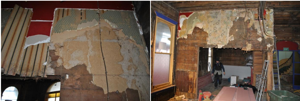
Plate 8: (Left) Layers of wall paper overlaying timber boards from the former Commercial bar of the 1887 ground floor. Plate 9: (Right) More layers of wallpaper on the sitting room of the 1901 Messenger layout.
