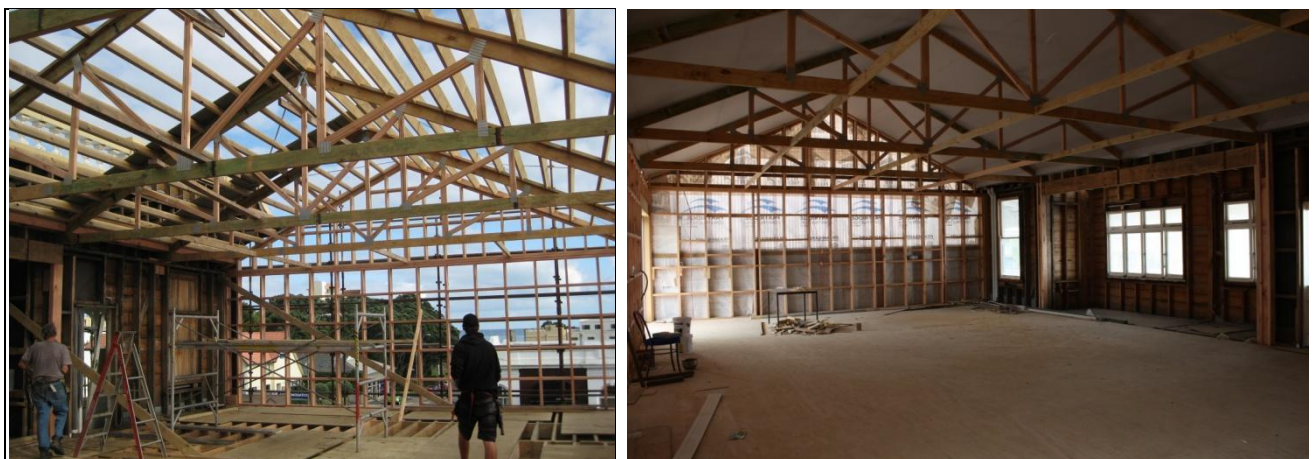
Plate 4: (Left) Demolished interior of the Messenger extension being rebuilt, street facade left standing.
