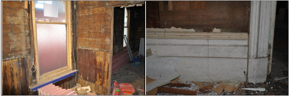
Plate 6: (Left) Polished rimu panelling in the former ground floor sitting room of the 1901. Plate 7: (Right) High skirting boards - detailed and made from a single board. From the 1887 dining room.
