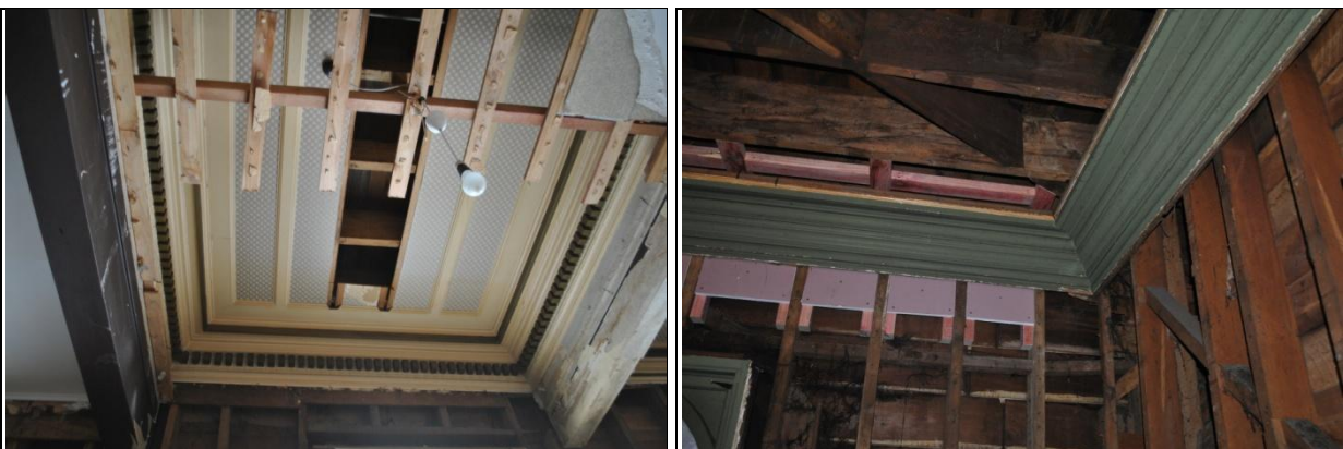
Plate 16: (Left) Ceiling of the Messenger extension to the dining room, exposed below a false ceiling installed mid 20 th C. Plate 17: (Right) Ceiling cornice above the main bar ground floor Devon St. The cornices in both plates have been retained in the refurbished building
