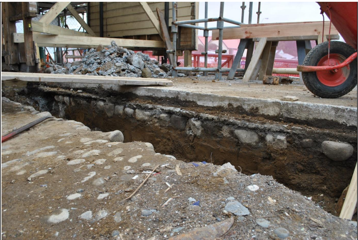
Plate 19: Cobbles exposed in section in foundation trench, overlying concrete was left in place following these works and subsurface cobbles remain unaffected
