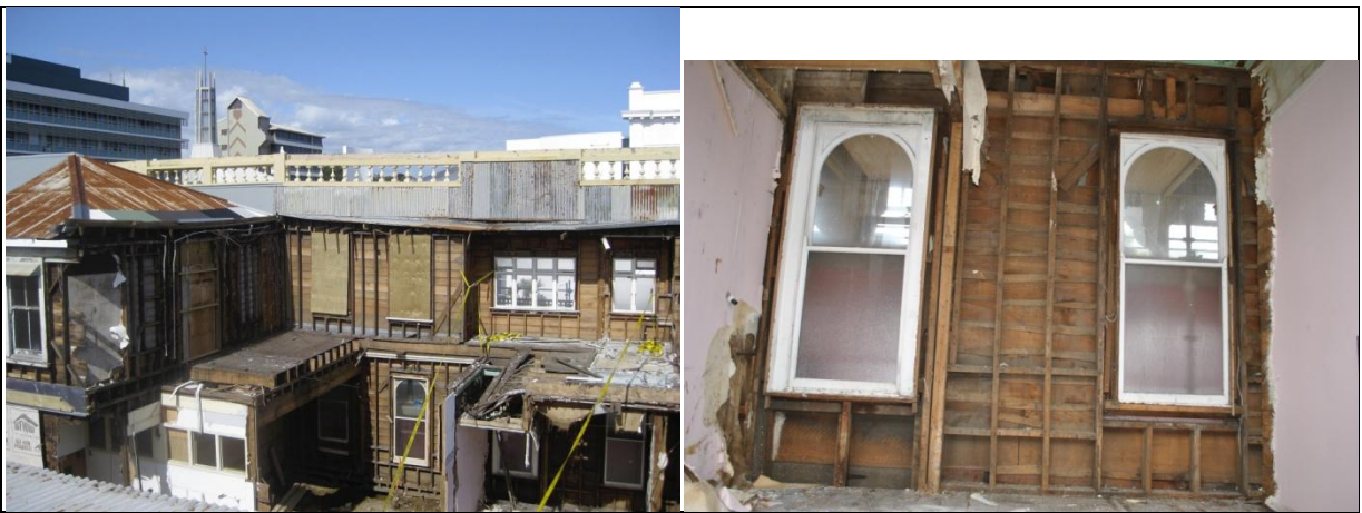
Plate 14: (Left) Interior view of the remaining Messenger extension facade with demolition almost complete. The 1887 Hotel remains standing and largely unaffected. Plate 15: (Right) Interior view of the exterior cladding of the Messenger extension, all weatherboards lapped at the joins on the interior using waste cuts trimmed from long boards.
