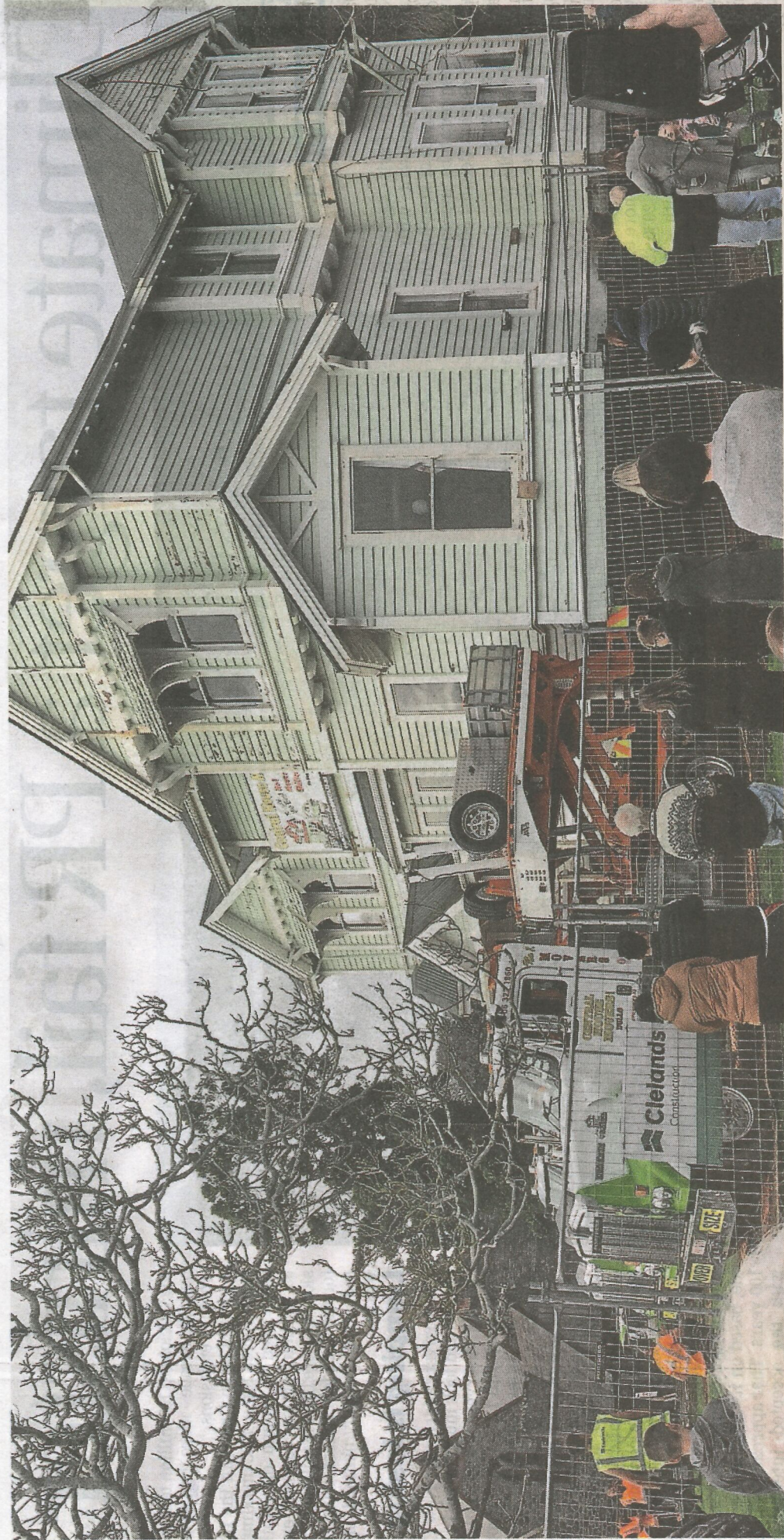
The vicarage at St Mary's was moved forward so it can be renovated.
