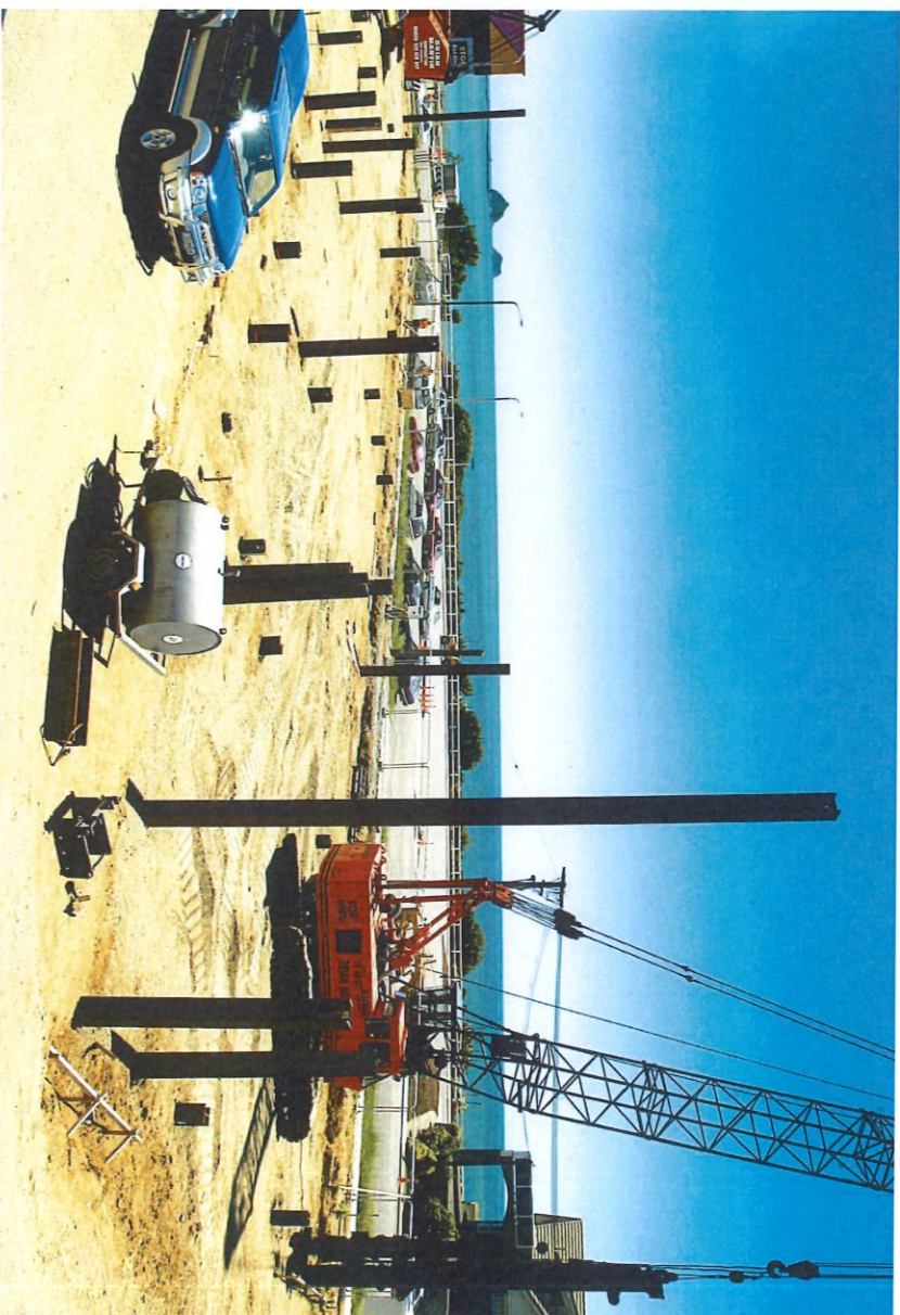
BUSY BASE: Construction of the Quarterdeck has started with site clearance and piling on the former Classic Fashions site. Photo: PIP GUTHRIE
