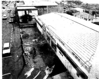
ON HIGH: Former bottle store premises are currently being converted into upmarket apartment accommodation.
